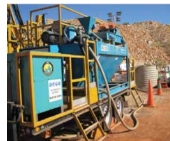
AMC Surface SRU™ on site.
